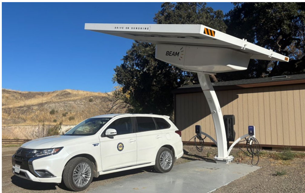
Figure 2-18: BEAM Global EV charger at the Altamont Sector office.
