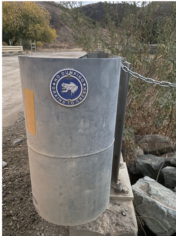
Figure 2-16: Example of installed storm drain marker.
