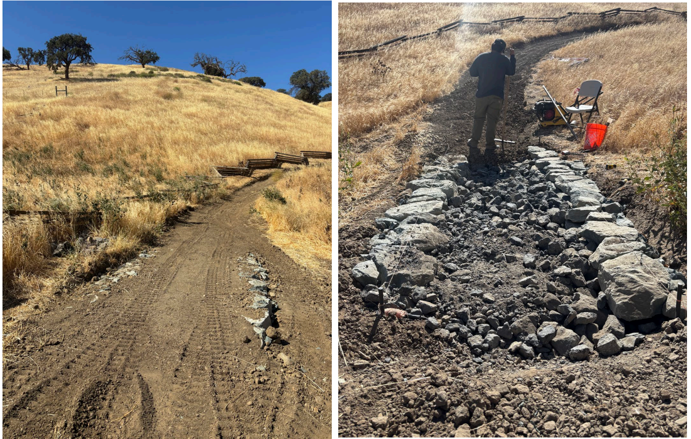
Figure 2-26: Drainage causeway installed in Harrison RMA.
