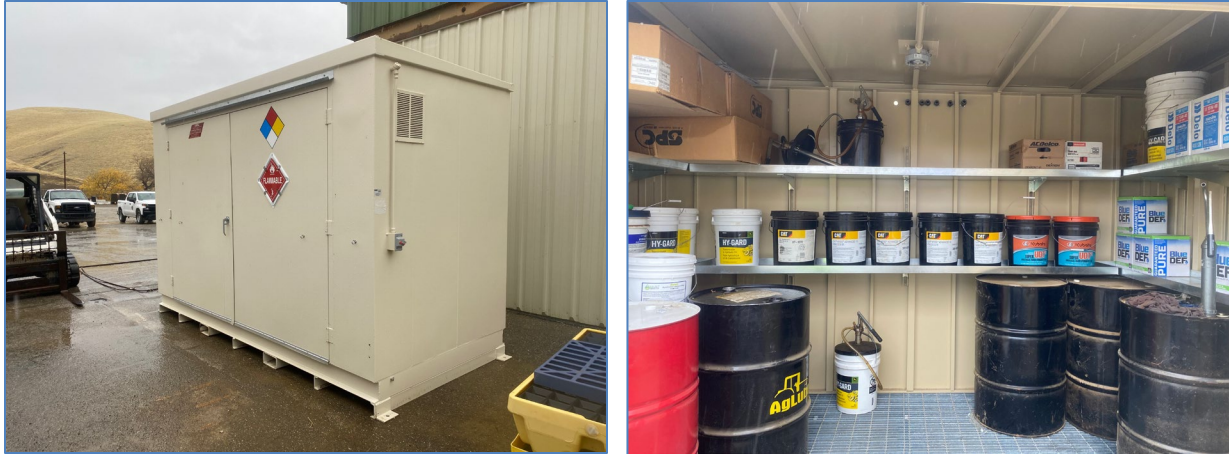
Figure 2-17: Oil containment system in the Carnegie SVRA Maintenance Yard.
